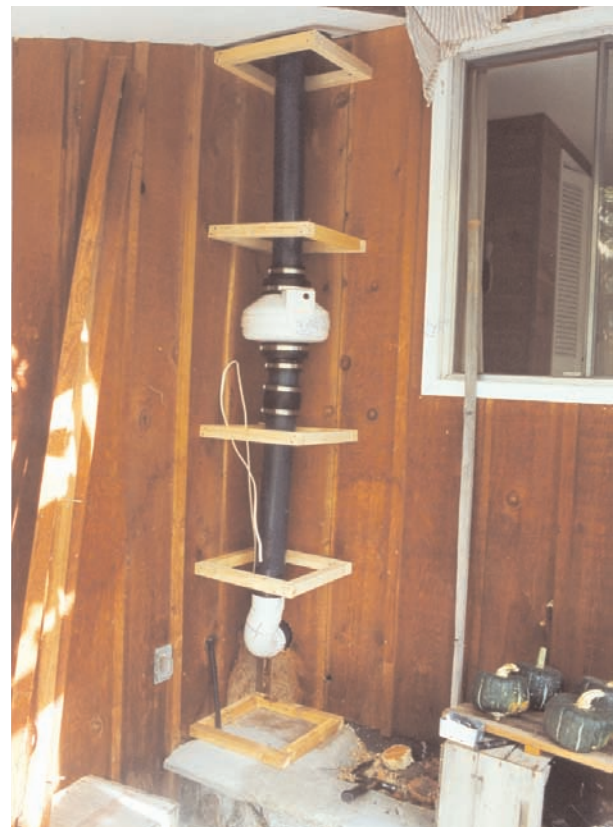
If a "passive" vent isn't enough, a fan can be added to pull the air outside the house.
